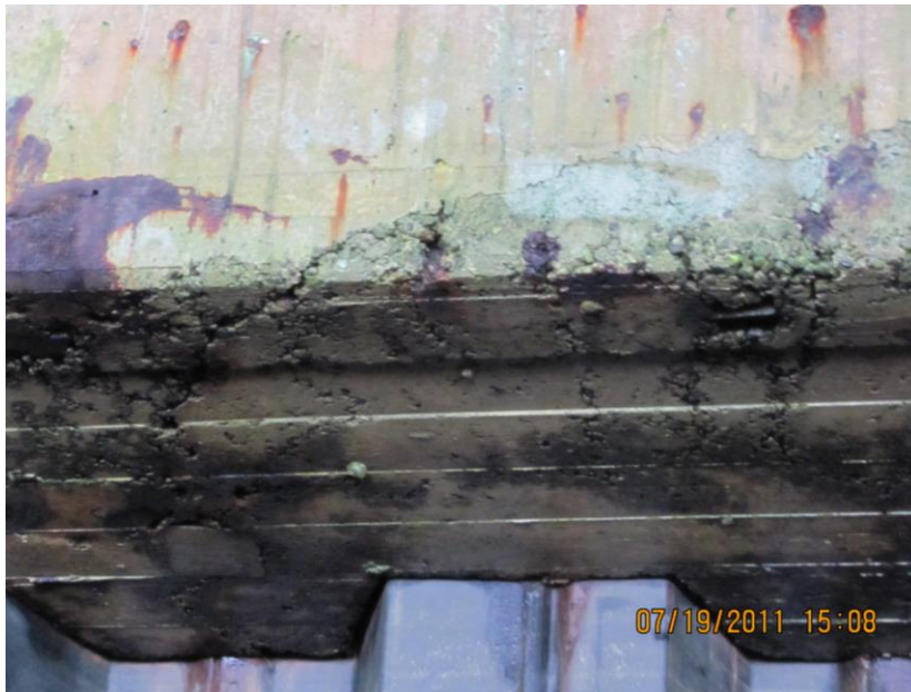
Sample Pile Cap Damages
