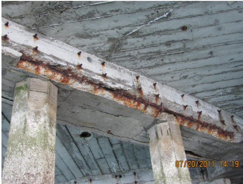
Sample Pile Cap Damages
