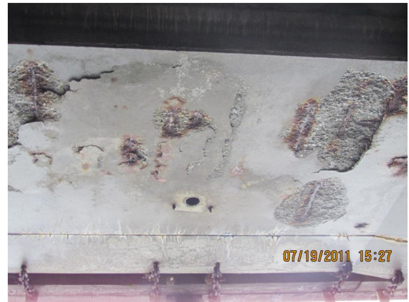
Sample Deck Panel Damages
