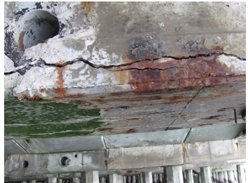
Sample Deck Panel Damages
